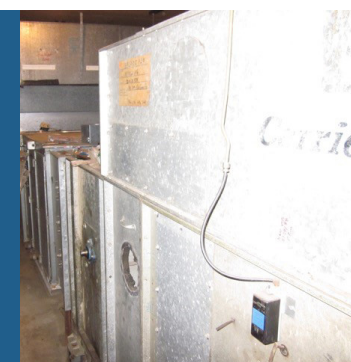
Portion of former HVAC system consisting of commercial boiler and chiller system
