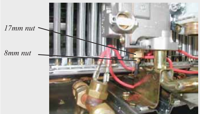
Electromagnet location (view from bottom of heater)
