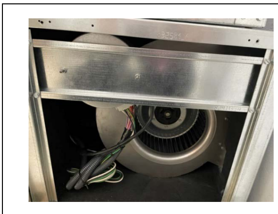
Fig.8 Final Installation, electrical harness connections facing down.
